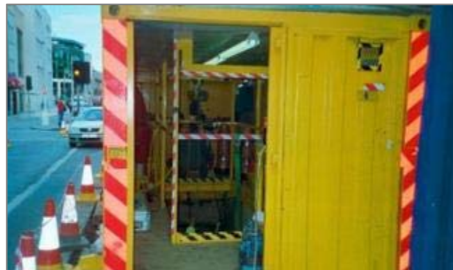
Figure 11 - HV cable jointing container
